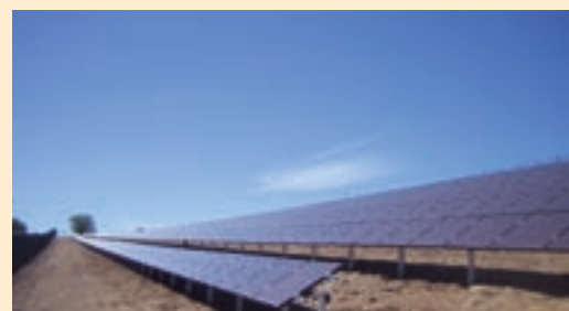
PV plant Lameelas, Portugal
